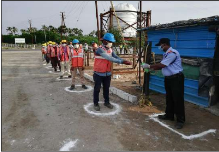
Hand Sanitizing facility at the entrance at Coal Jetty Project Site, TANGEDCO, Udangudi, (45418 DM)
