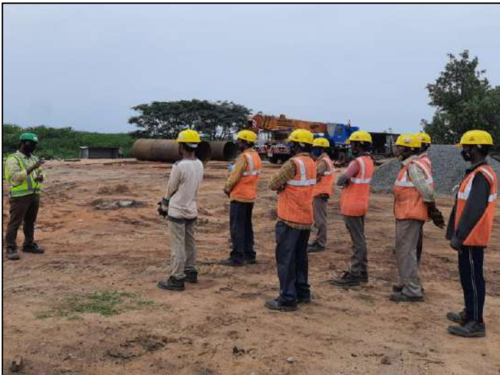
Social Distancing maintained during TBT at Liquid Jetty Site KPCL, Krishnapatnam, Andhra Pradesh (49520 DM)
