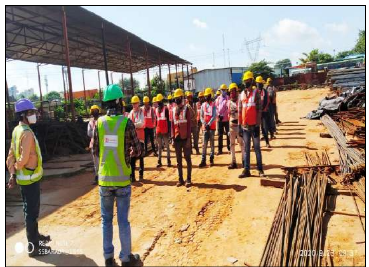
Daily Toolbox Talk conducted on Covid-19 Precautions at A1717BW/ D2 (BMRC -R1B) Project site.
