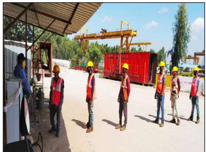
Regular Thermal Temperature monitoring being done at A1717BW/ D2 (BMRL R1B) Project Site
