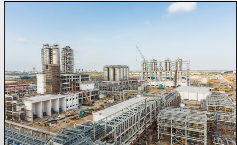
Paradip Refinery – Industrial Complex
